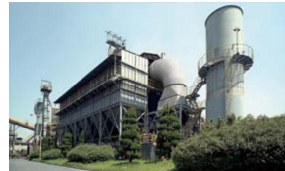
Electric Precipitator for Blast Furnace No. 5, Gwangyang Works, Korea
